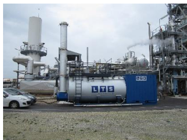
An LTS steam boiler
