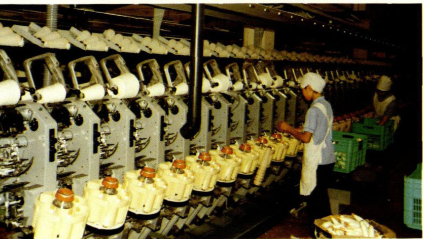
China's second largest cotton mill uses oil-free compressed air at all stages of the production process.
