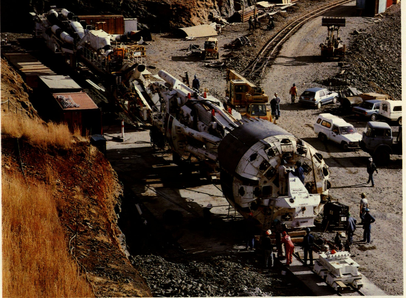
Robbins tunnel-boring machine (TBM) is made ready for boring a section of the major hydro power plant project in Lesotho.
