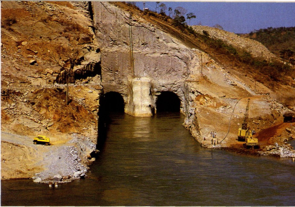
Two Atlas Copco jumbo rigs were used for tunnel boring work at the Serra da Mesa power station project, in Brazil.
