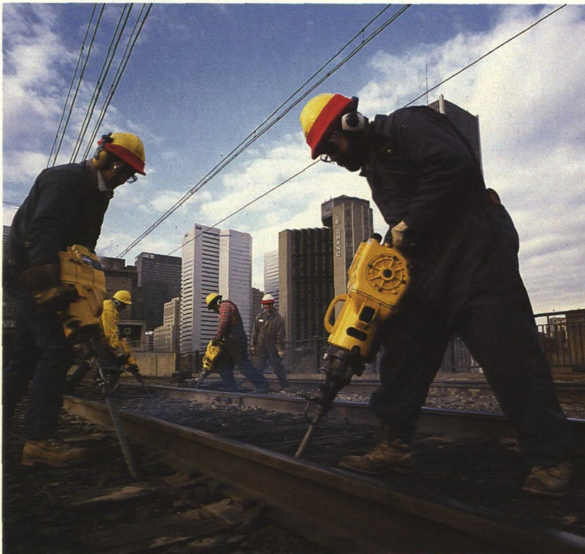
CNR, Canadian National Railways, regularly uses the Pionjär fuel-powered drill for compaction work.
