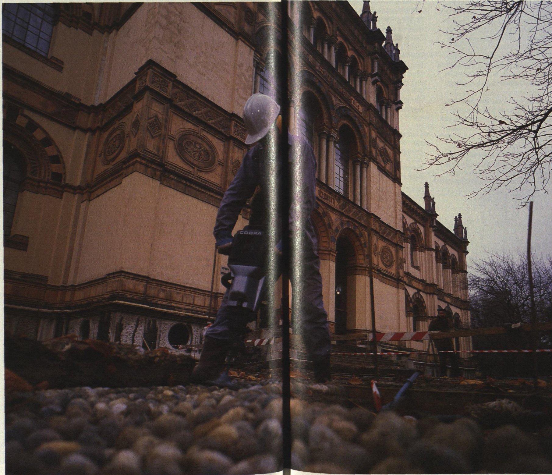
Laying pavement stone in Milan, Italy, is one of the many tasks handled by the Cobra, a fuel-powered portable drill/breaker. It is also used for rock drilling, breaking, light compaction and digging.
