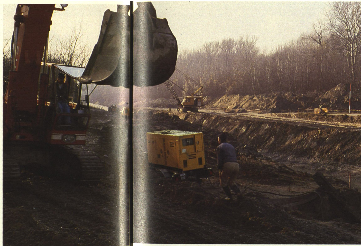
Diesel-powered generators were introduced during the year to provide mobile sources of energy at construction sites. The generators are used for lighting, welding, pump operations, power drills and other tools. The generator pictured is being used as a power plant on the Austrian section of the natural gas pipeline being built between the Soviet Union and Italy.
