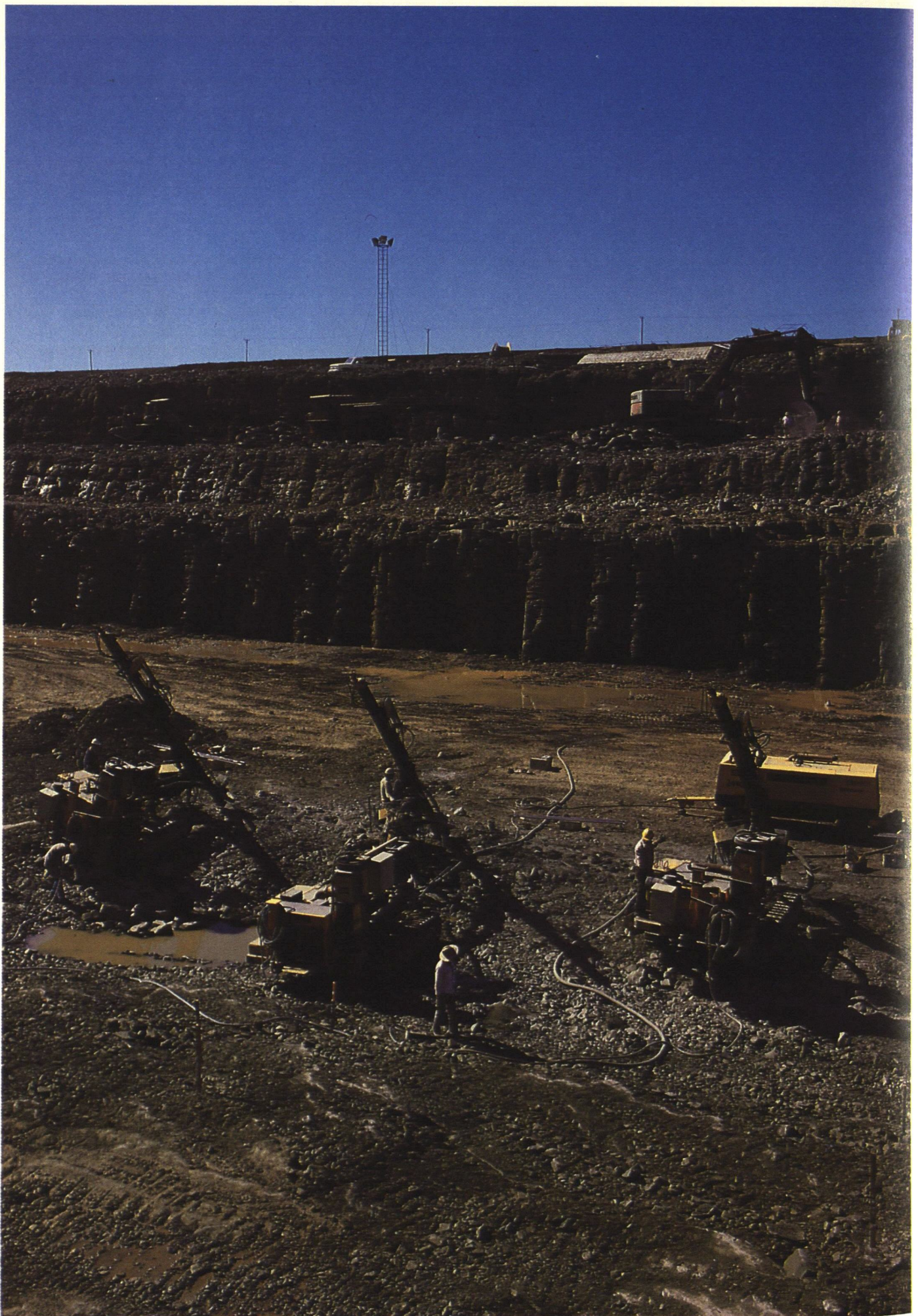
Impregilo, an Italian Contractor, selected Atlas Copco to supply the rock drilling equipment for the Yacyretá hydro power project in Argentina, which involves construction of one of the world's largest dams.
