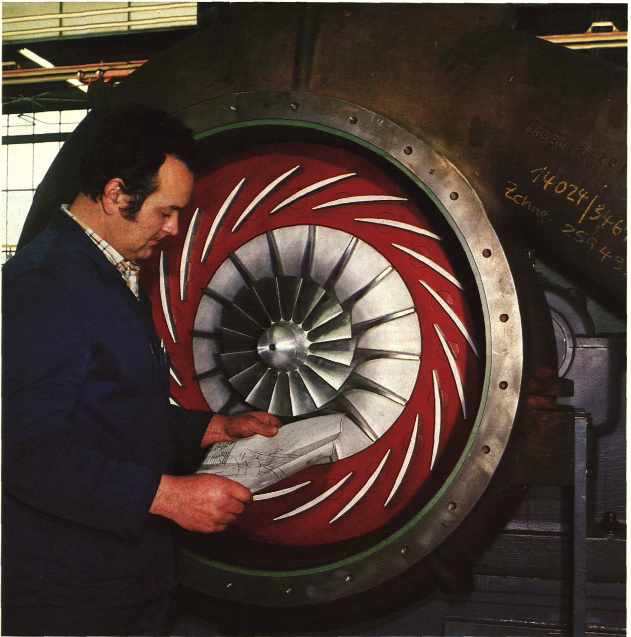
Installation of a turbo compressor at the Atlas Copco Energas factory in Cologne. This is a new technical area being offered on the world market by Atlas Copco.
