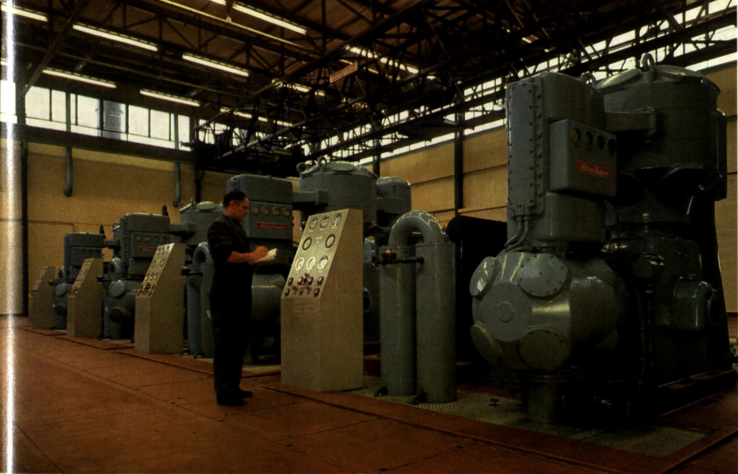
Part of a modern compressor installation plant at one of Vauxhall Motors' manufacturing centres in the U.K.
