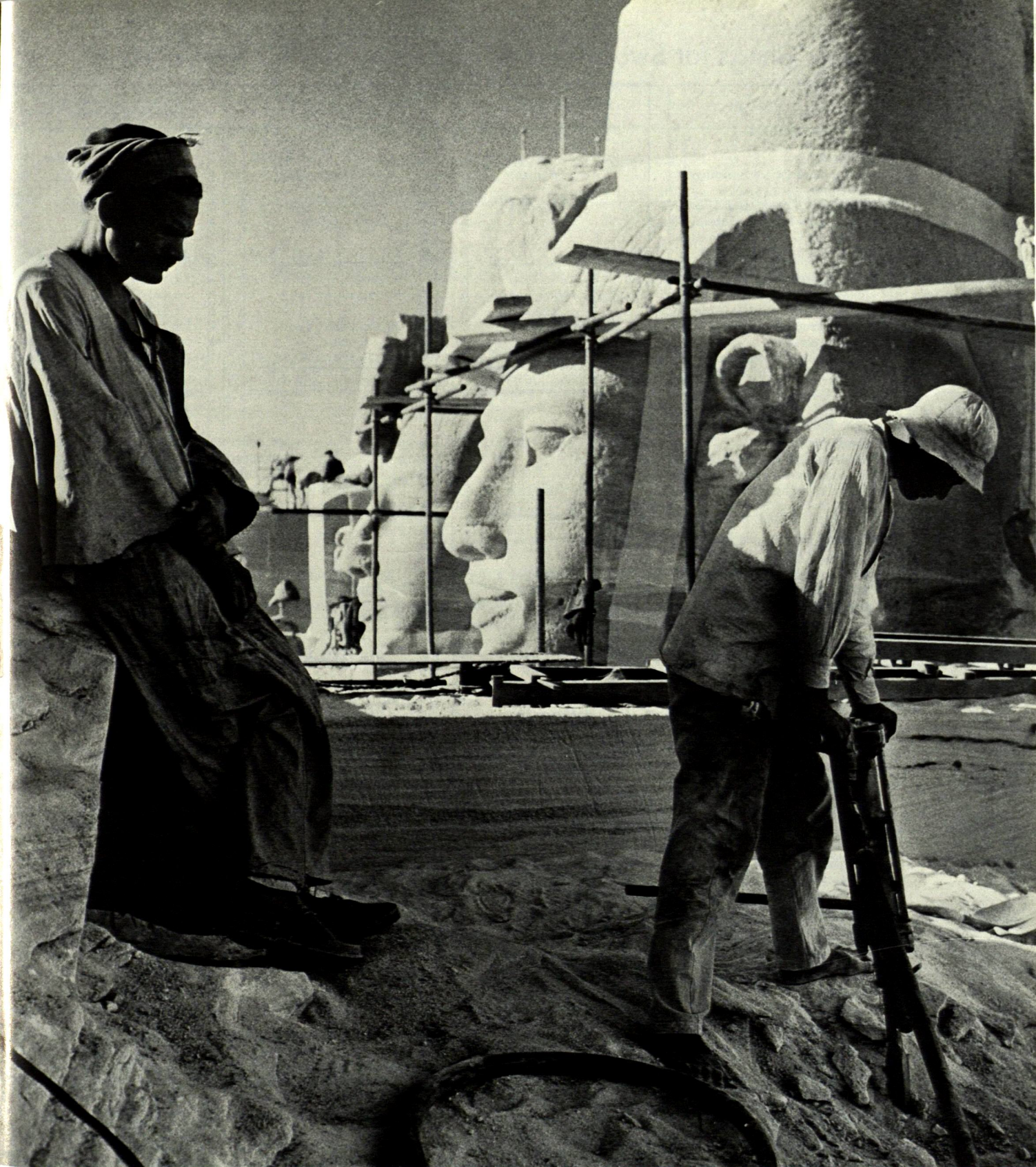
The Abu Simbel temples, carved out of the sandstone flank of the Nile 3,200 years ago, have attracted the greatest interest of the Nubian monuments being saved from the rising waters created by the new Aswan High Dam. More than 100 TEX breakers are included in the Atlas Copco equipment used by the international consortium of contractors for the project.
