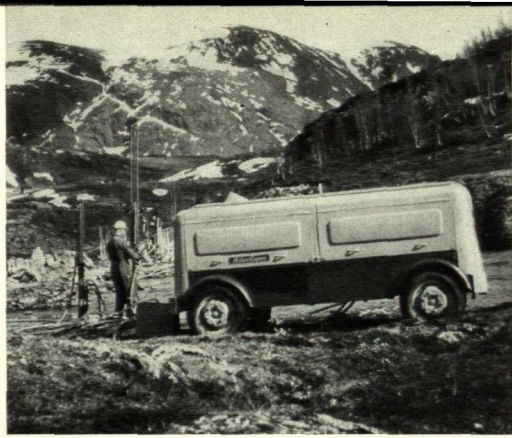
Drilling for initial blasting on a large hydro-electric project in Norway. A "Twin-Air" screw compressor operating two Atlas Copco "Bencher" drilling units.
