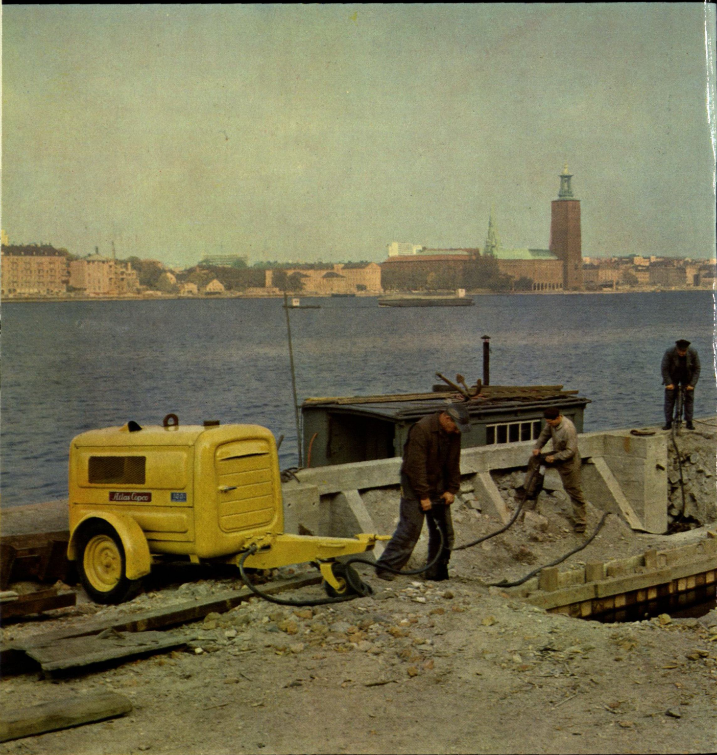
A Stockholm working scene: an Atlas Copco VT4 compressor powering new E-type breakers on a harbour repair project.
