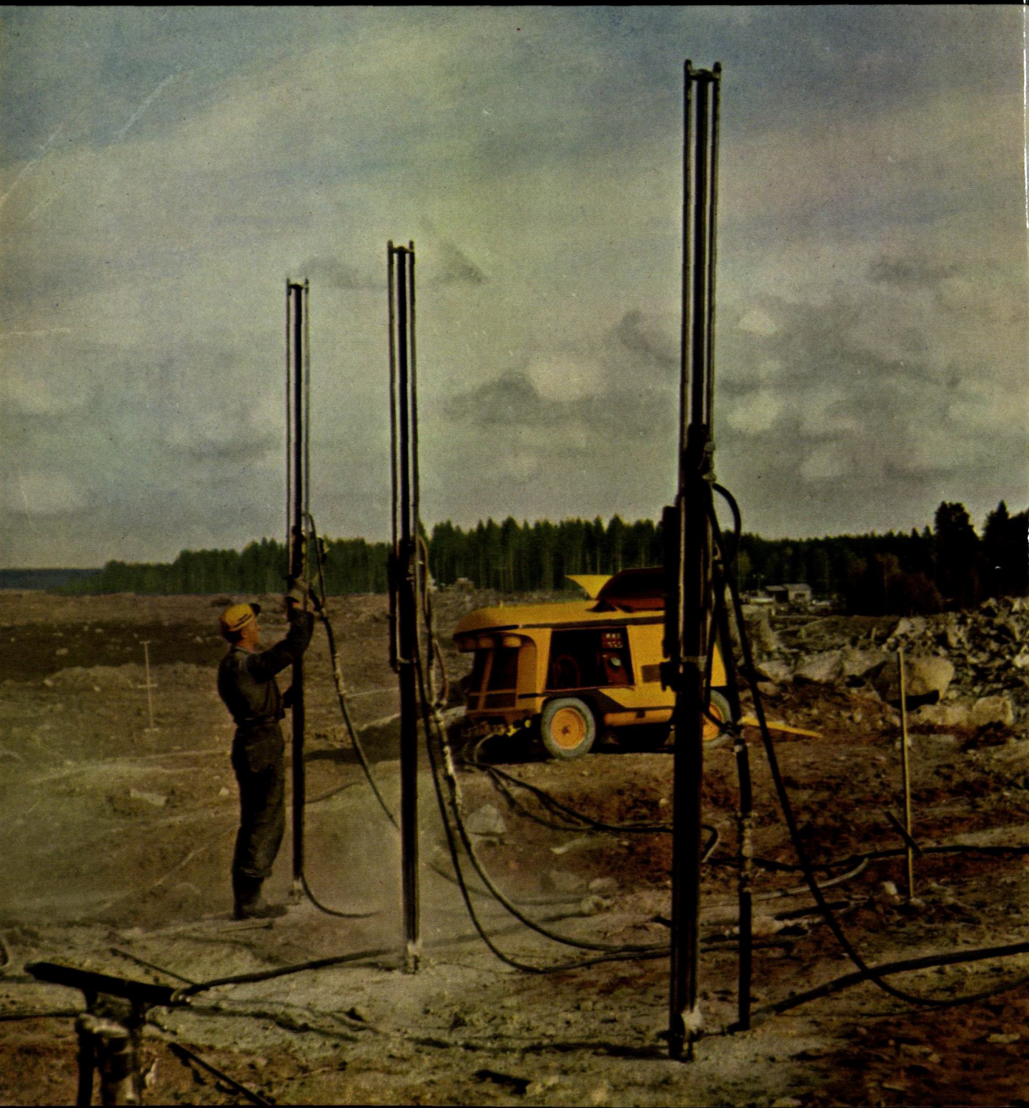
A "Twin-Air" rotary screw compressor operating three "Benchers"—Atlas Copco's new rock drilling equipment—at Arlanda, where Stockholm's jet age airport is being built.
