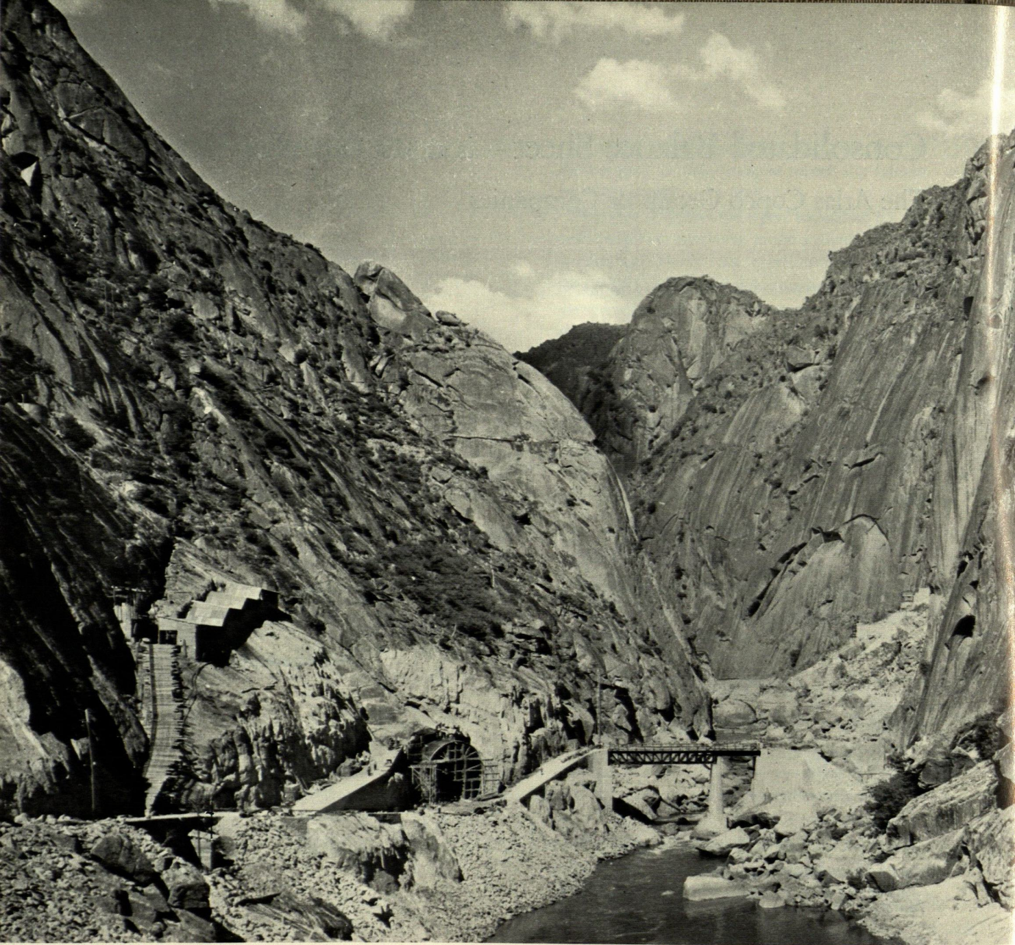
The photograph above shows Salto de Aldeadávila in Spain, where the largest water power station in Europe is being built, and where tunnelling operations are being carried out with Atlas Copco equipment.
