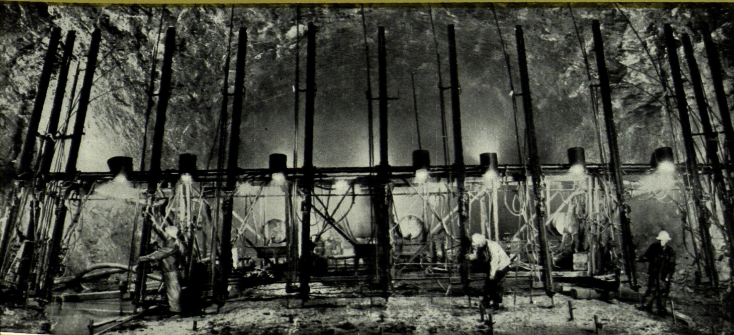
When excavating the world's largest tunnel at the Stornorrhors, Sweden, 500 feet per manshift were drilled with Atlas Copco chain-fed drills.
