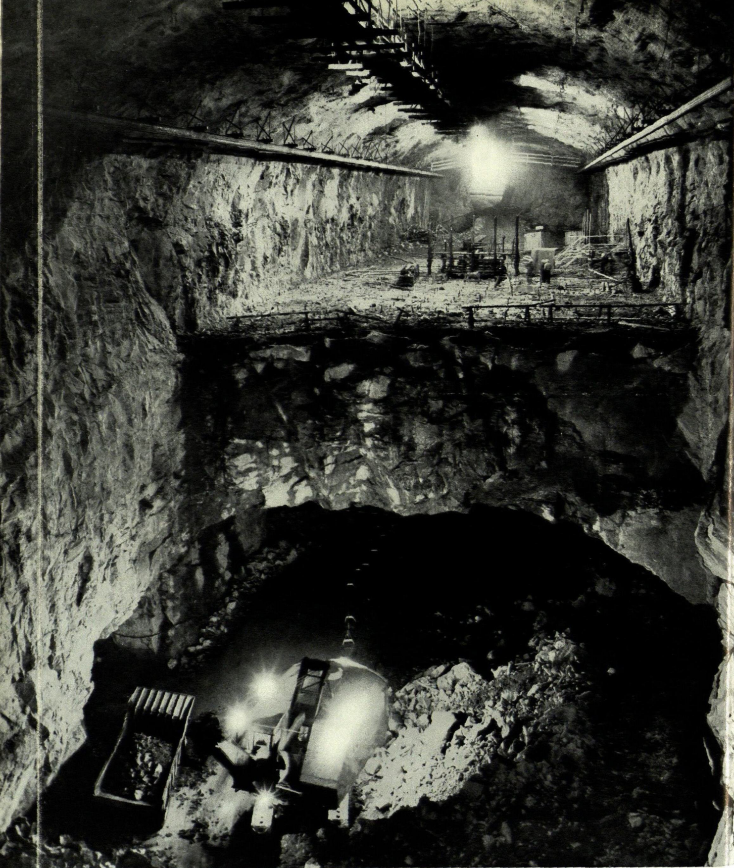
At Stenungsund the Swedish State Power Board are using Atlas Copco drills and compressors in the construction of the vast rock chambers needed for a new steam power station.
