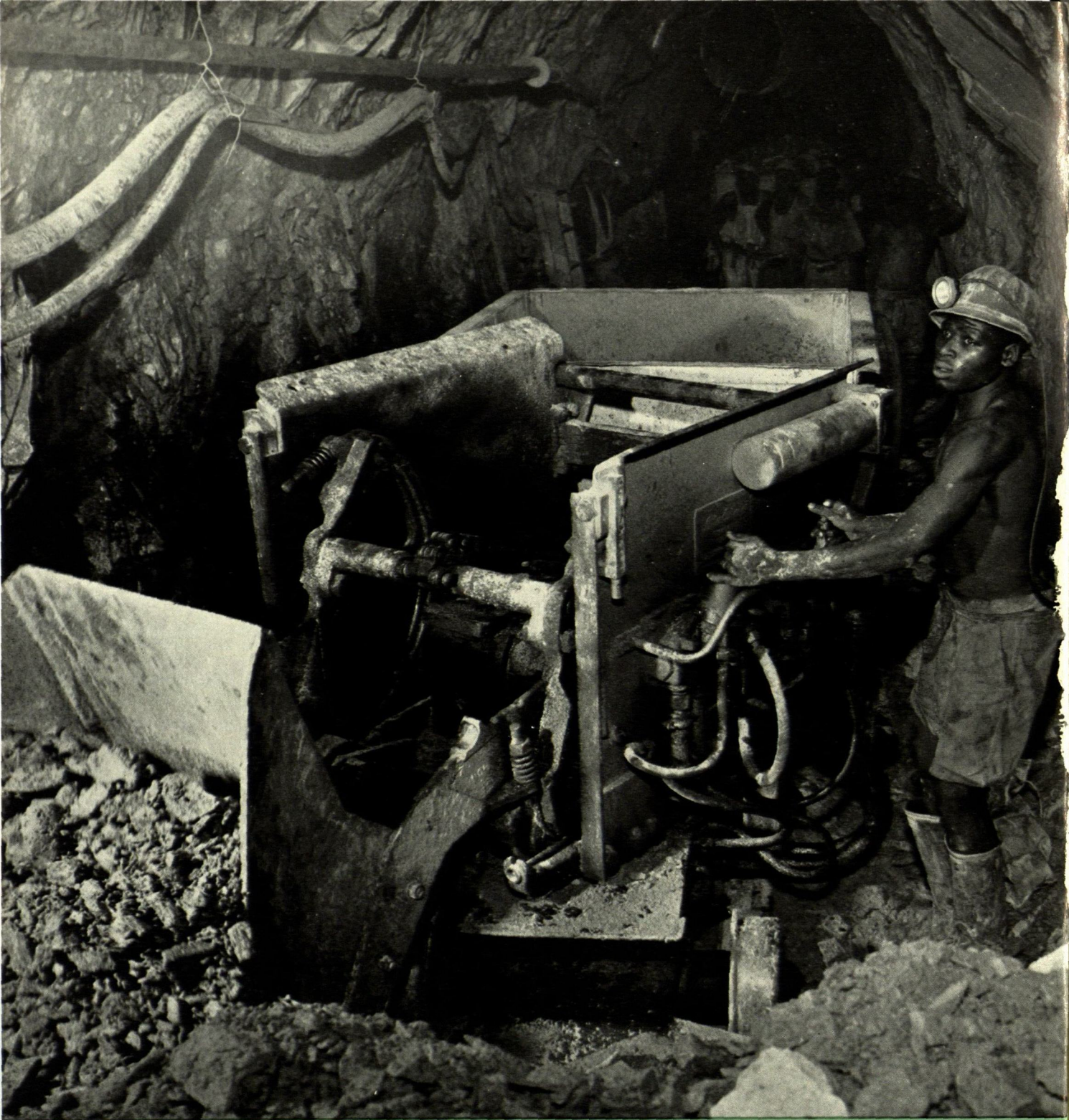
A pneumatic loader, type LM 100, at a depth of 15,750 ft. in the South African gold mine Durban Roodepoort Deep.
