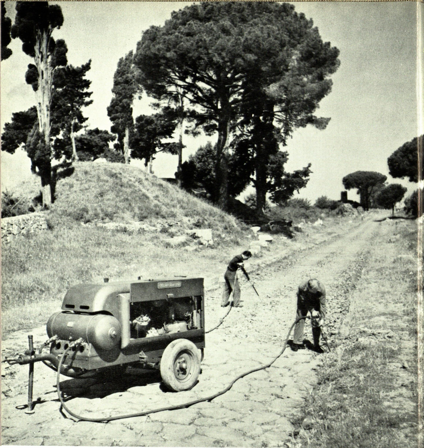
Italy is one of the countries in which Atlas Copco has effected greatly increased sales. The photograph shows a portable compressor and two pneumatic paving breakers being used in restoring the Appian Way, an old Roman military highway.
